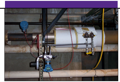
Rosemount Orifice Plate (check meter) installed downstream of the Rosemount Compact Orifice Mass Flow Meter.
